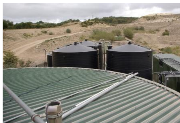
Figure 2 Biological tanks (in background) at Beacon Hill, providing three stages of nitrification, viewed from the leachate balance tank
