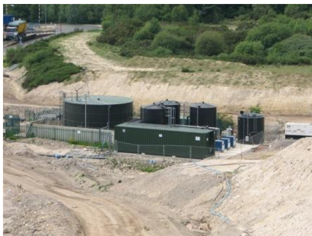
Figure 1 Wehrle containerised MBR/NF installation at SITA's Beacon Hill landfill site
