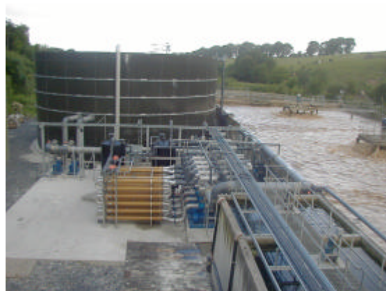
Dairygold BIOMEMBRAT adjacent To a conventional activated sludge plant
