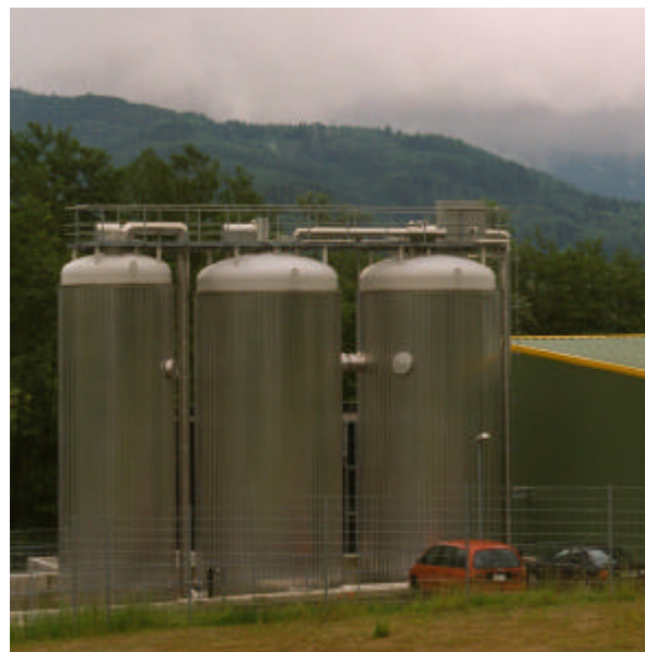
BIOMEMBRAT treating landfill leachate at Lorrach
