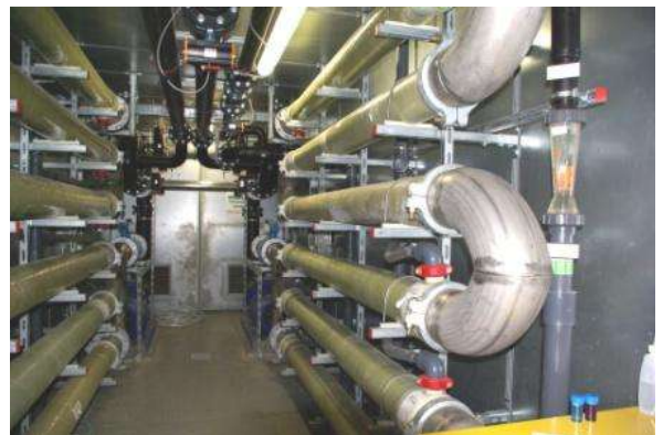
Figure 1 Wehrle containerised installation
