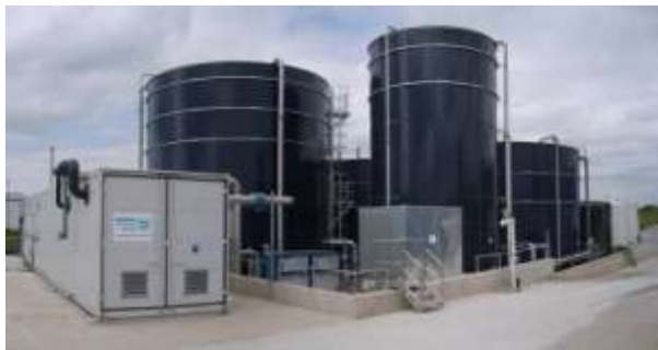
Figure 2 – Wehrle Wastewater Treatment System at Foston
