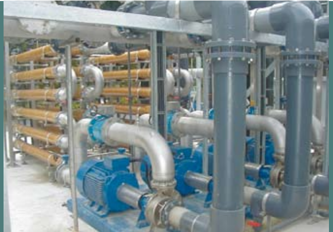
Figure 4 UF membrane system
