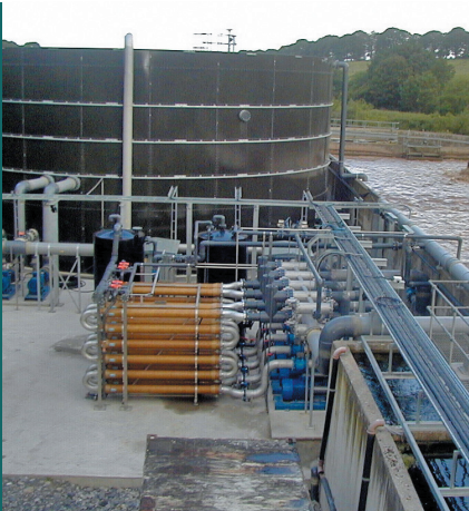
Figure 1 MBR Plant (before building erected) alongside second stage aeration basin
